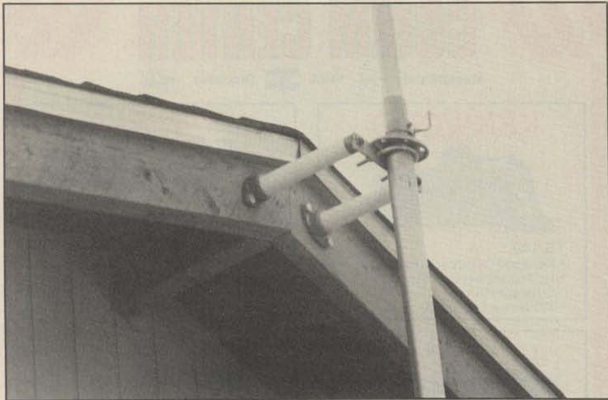
A simple, neat installation via long stand-off insulators.
